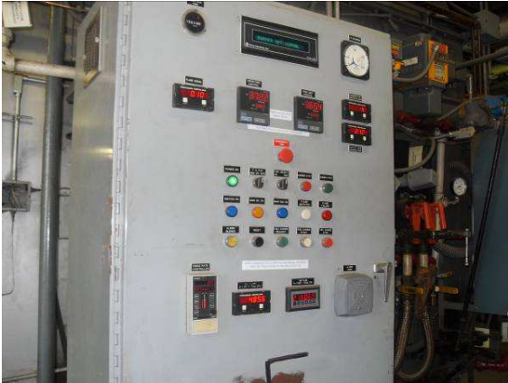
Control box for one of the three turbines
