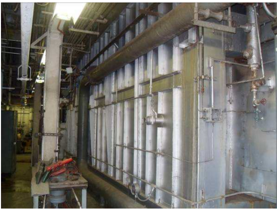
Side of the turbines
