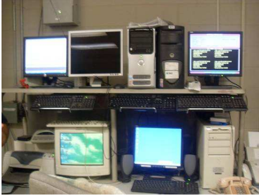
Figure 2.2 These are the computers that supervise the emissions of the plant. If the values do not meet the standards set by the federal government, the computers will alert the staff at the plant.
